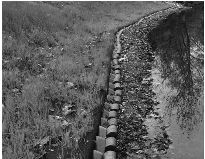
Fabric shall have the proper overlap and be free of any holes or tears.
