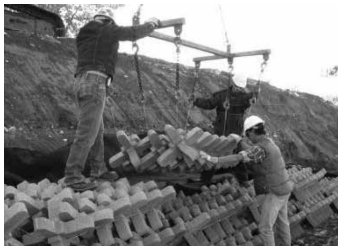
A spreader bar is essential to distribute the load without crushing the interior units.
