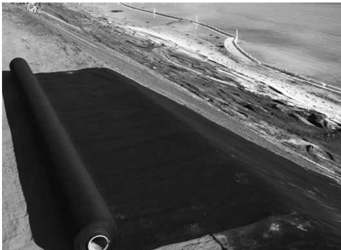
Geotextile filter fabric is placed directly on prepared subgrade and should not be disturbed.
