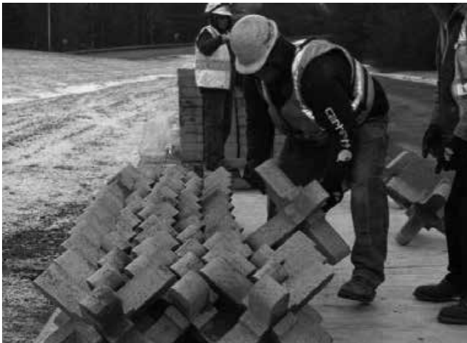
Bundling is required where the ability to set individual units is restricted.
