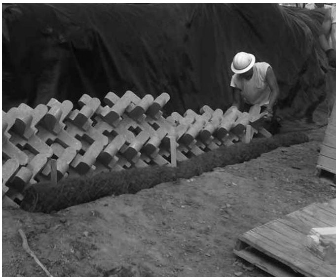
Proper installation of A-Jacks is important to achieving the intended hydraulic performance.
