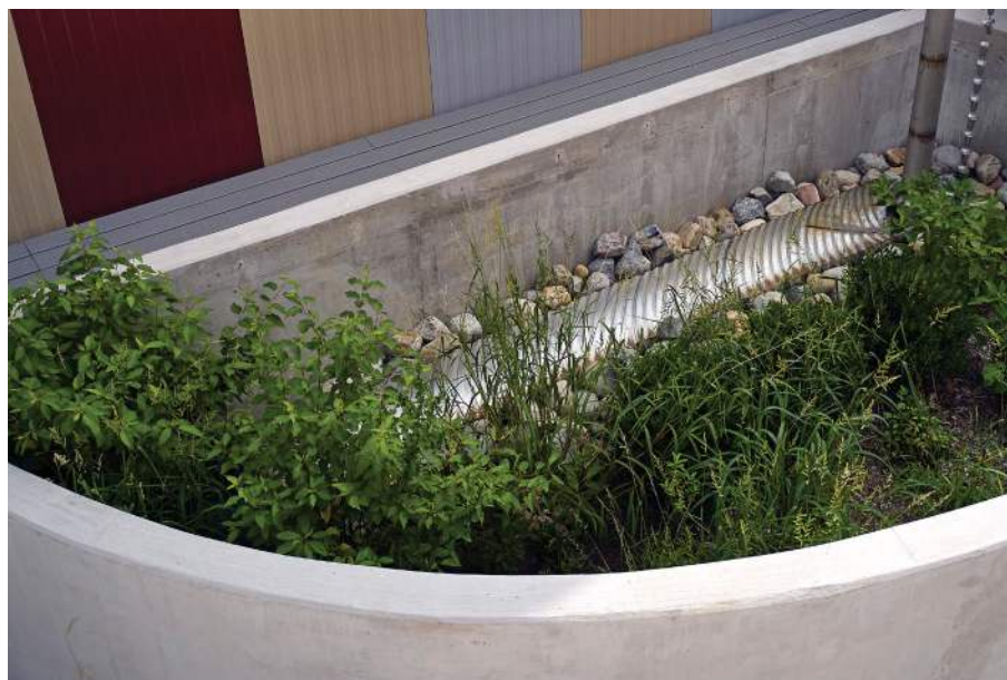
Inside view of the planted FocalPoint biofiltration planter box system.
