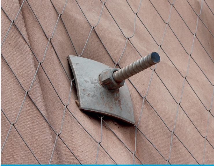
Rock bolt and large anchor plate with radiused corners
