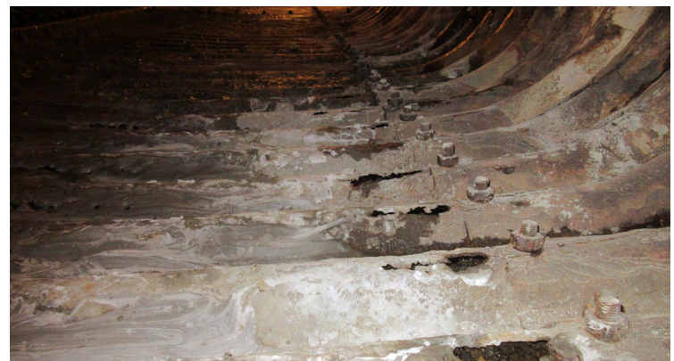
Filling of corrugations covering damage
