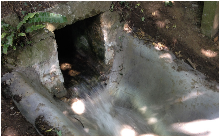
A suitable mortar can be used to join and seal CC to existing infrastructure
